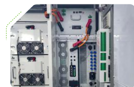
Energy storage cabinet
