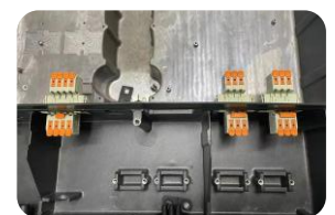
Energy storage cabinet
